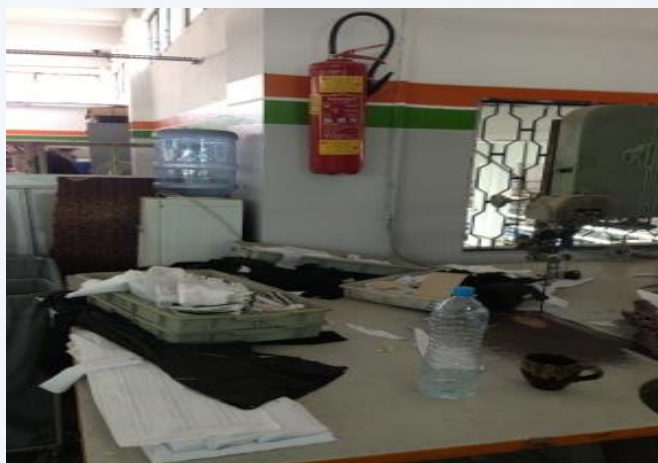
Some extinguishers were found obstructed during the assessment
