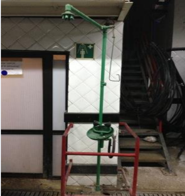
This emergency shower is not well installed and not connected to water
