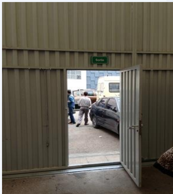
The main fire exit door is narrow and opening inward
