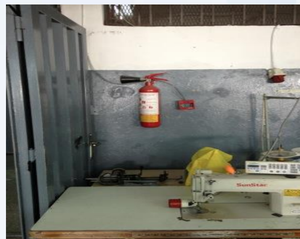
Fire alarm + Extinguisher with no identification sign + obstructed
