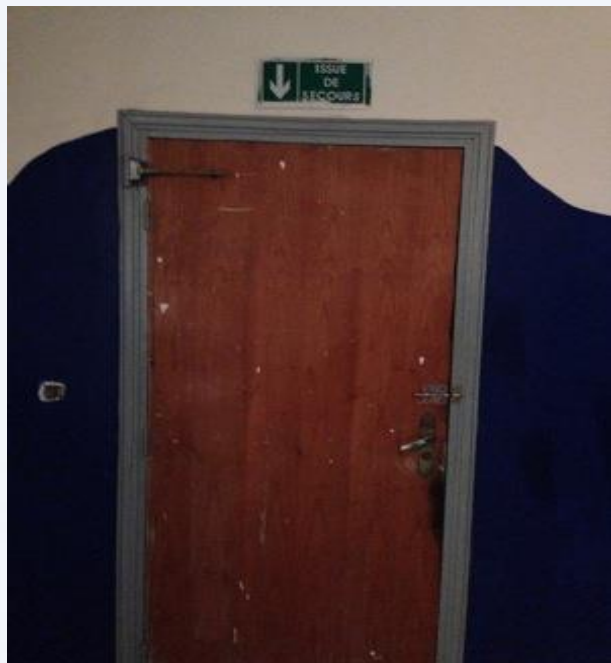
Fire exit door found blocked during the assessment
