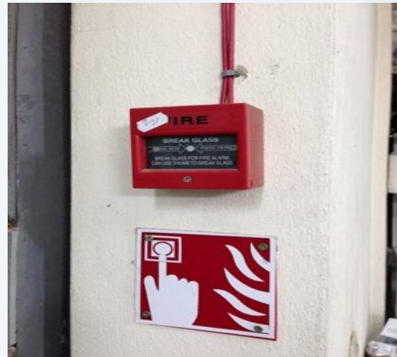
Fire alarm is available and well-identified
