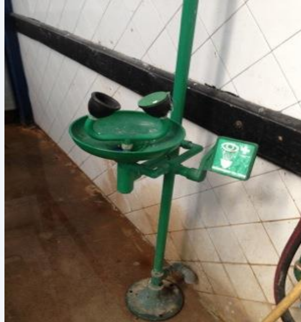
Eye shower installed in chemicals manipulation area but it's not operational
