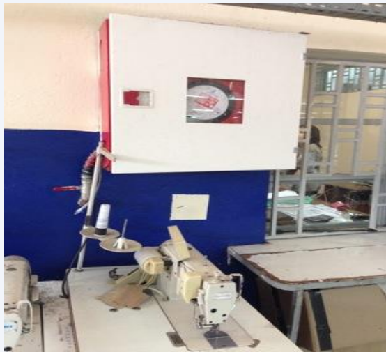
Some fire hoses were found obstructed during the assessment
